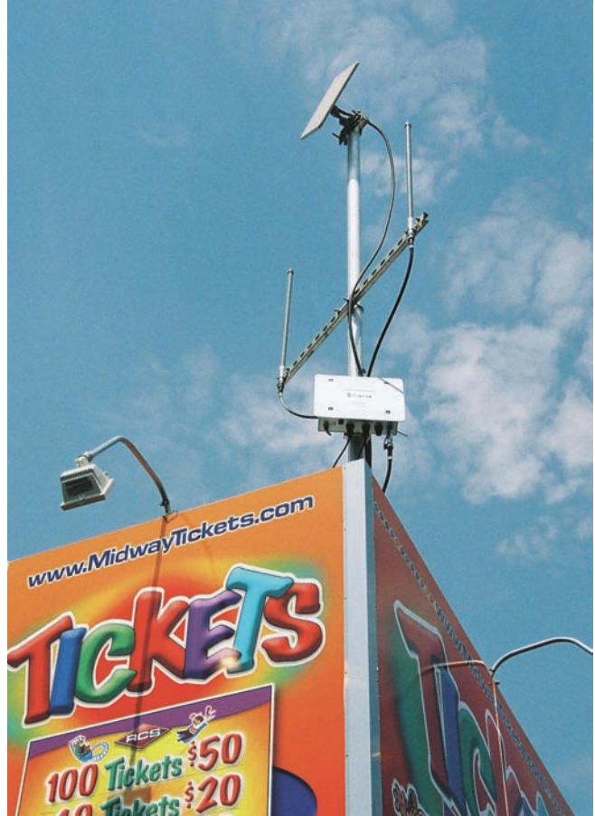
Firetide node installed on a ticket booth
